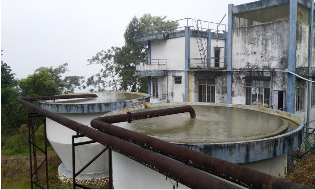
Photo plate 3.5: Sedimentation Tank at Water Treatment Plant near Tuipui Pump House-II.
