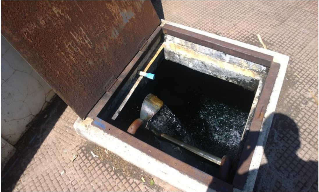
Photo plate 3.9: Site 2- Inlet of filter water at Darthlalang tlang main water reservoir.
