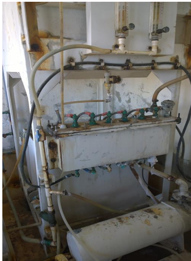
Photo plate 3.10: Site 2- Chlorinator unit for disinfection of water at Darthlalang tlang.
