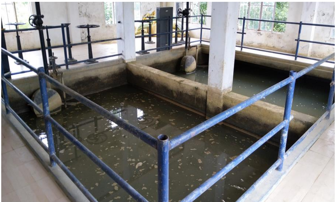
Photo plate 3.6: Filtration Tank at Water Treatment Plant near Tuipui Pump House-II.
