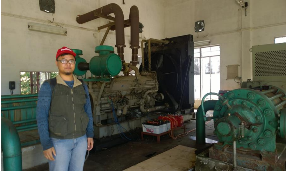
Photo plate 3.7: Water pumping unit located at Tuipui Pump House-II.
