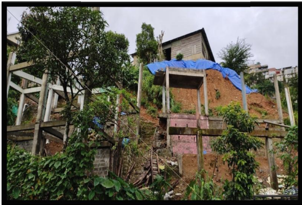
Fig. 3.8 : Houses dismantled by landslide at College veng locality, Lunglei
