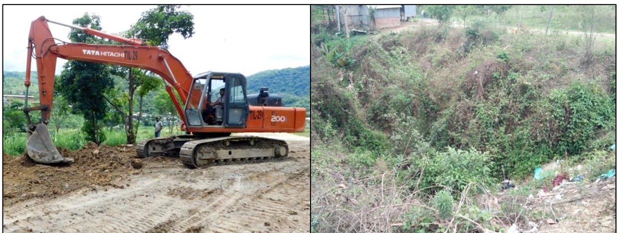
Photo 9: Excess soil and waste dumped on nearby ditches.
