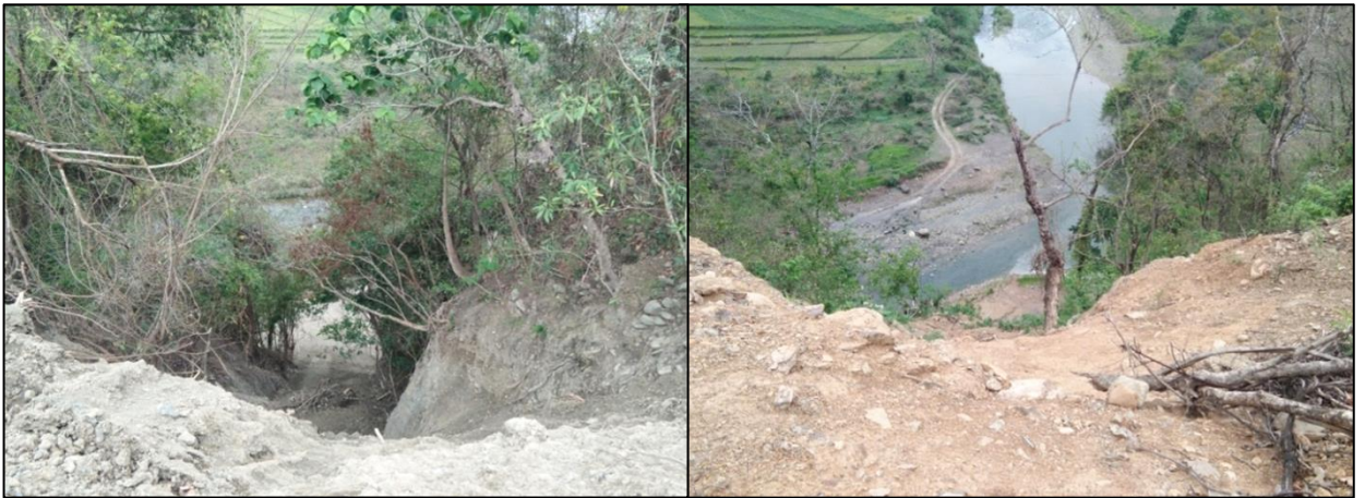
Photo 8: Excess soil from slope cutting deposited in the Tiau river.
