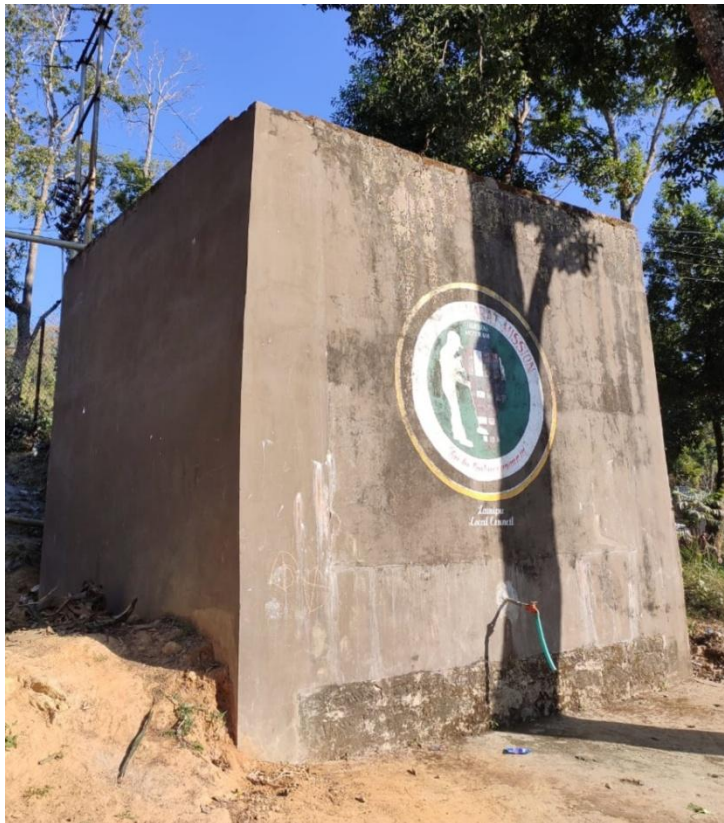
Photo plate No.14: Large water tank at Lawipu. Source: Site visit
