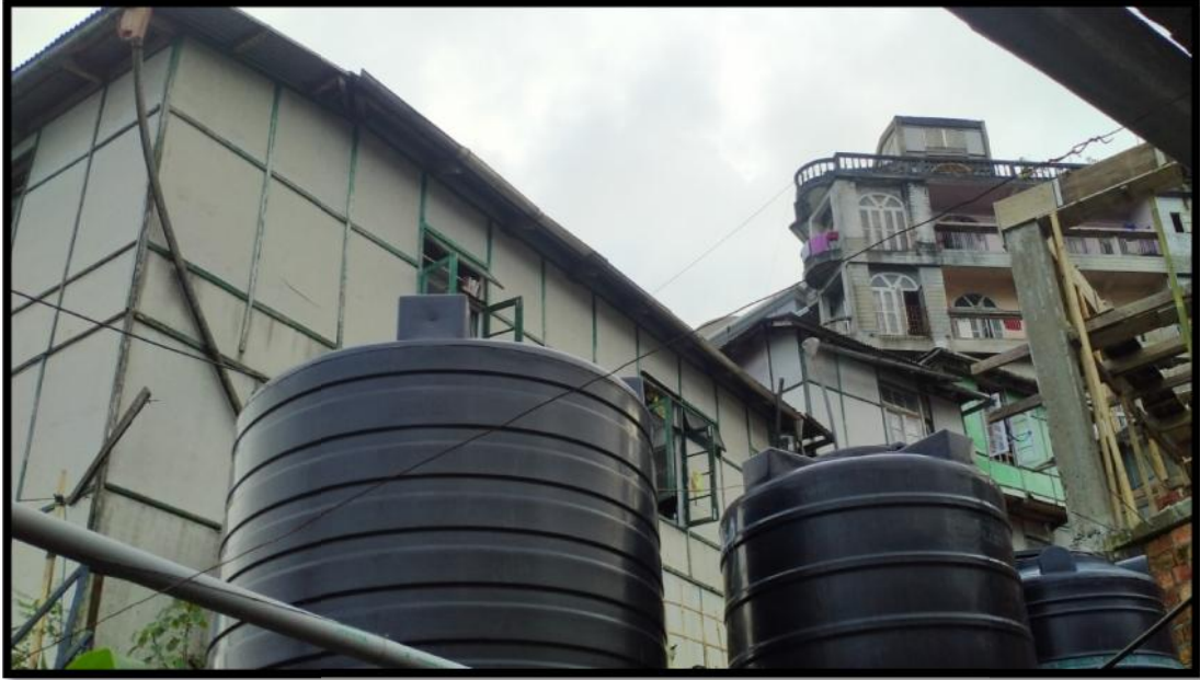
Pics: Rooftop rainwater harvesting in Aizawl city.
