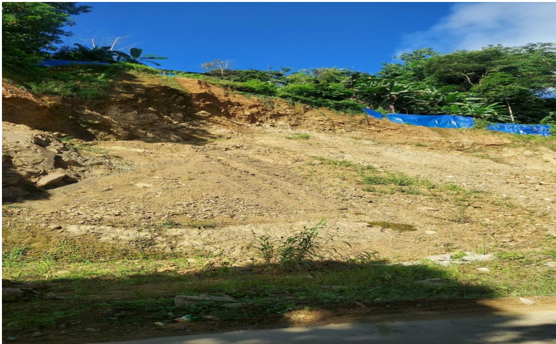
Location 8. Landslide (Translational type) near National highway, Melriat.
