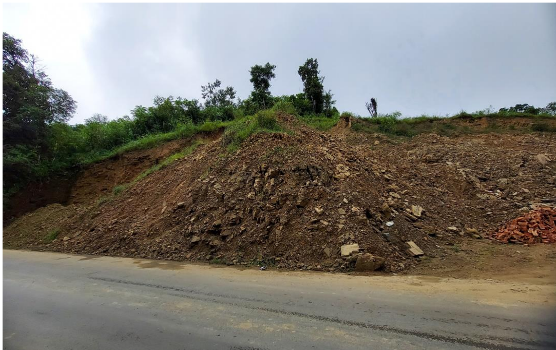
Location 14. Landslide (Translational type) near national highway, Chamring.
