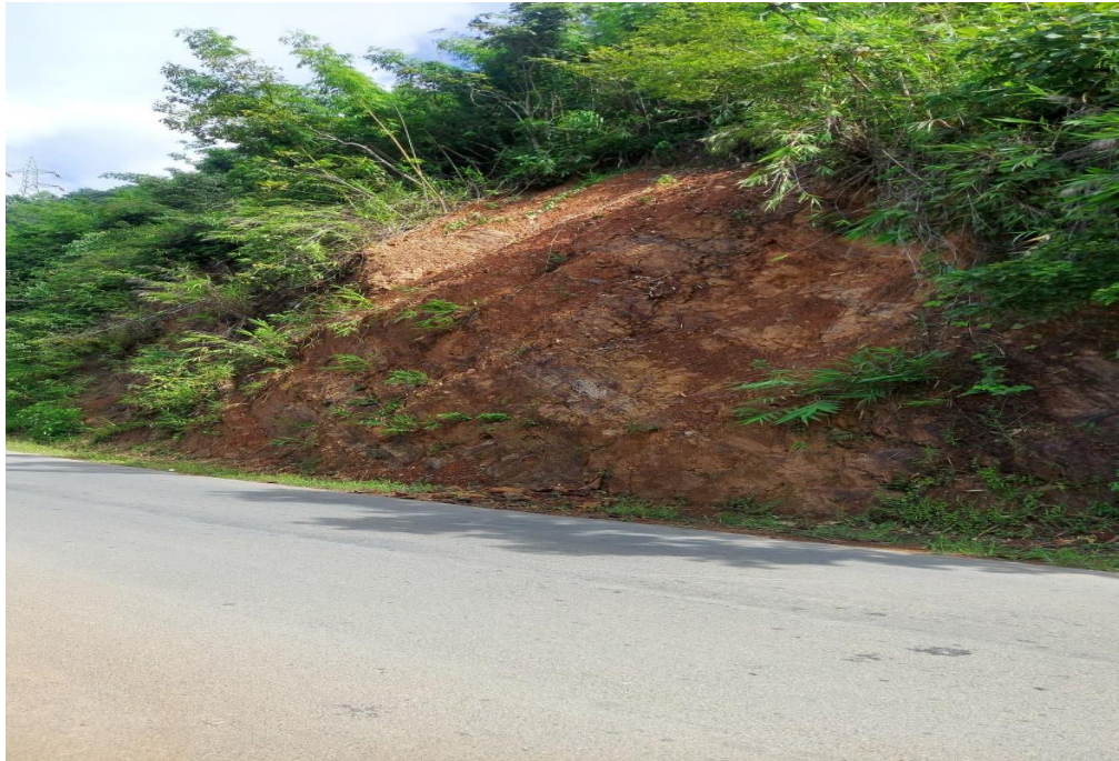
Location 9. Landslide (Translational type) near National highway, Tachhip.
