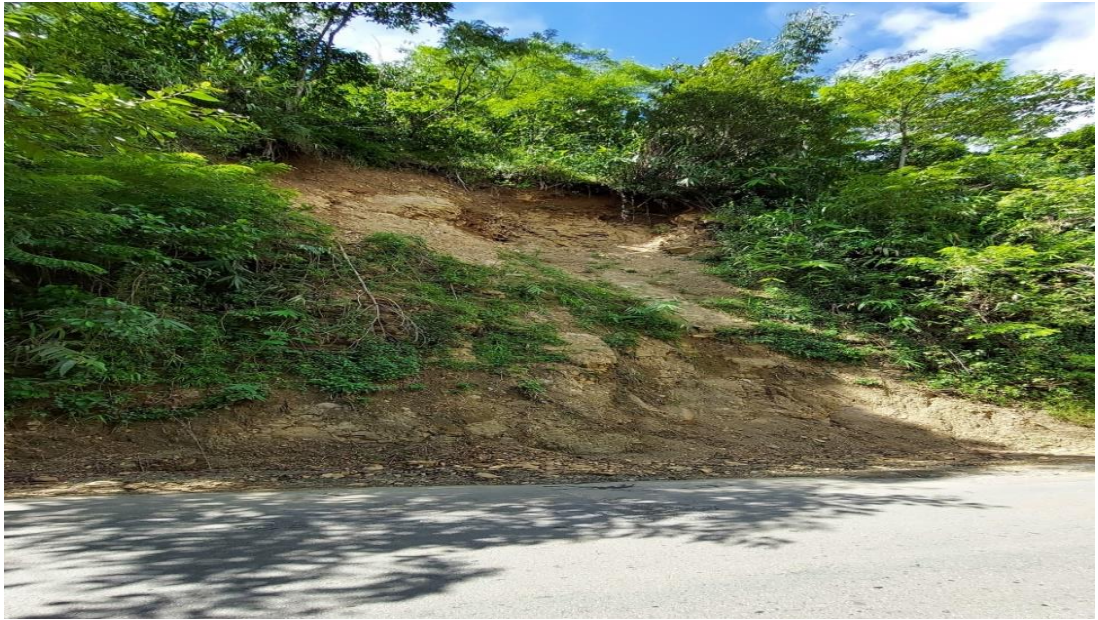
Location 17. Landslide (Translational type) near national highway, Sialsuk.
