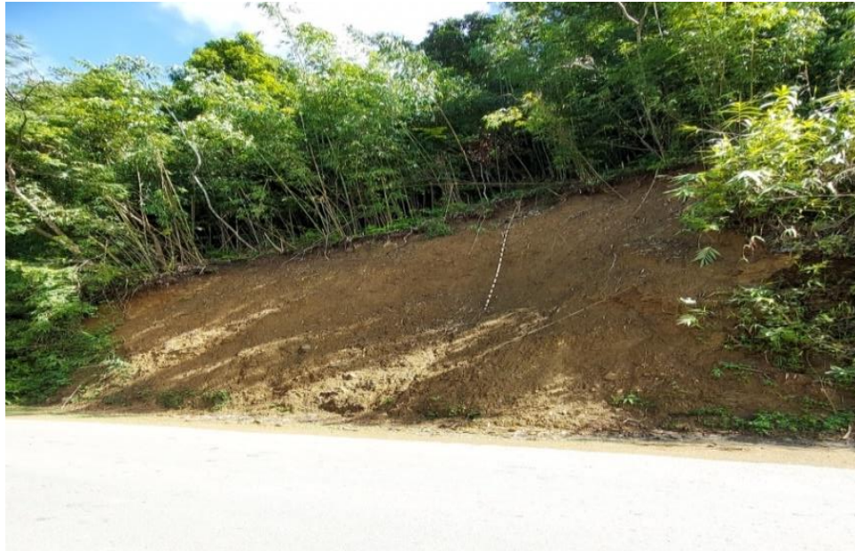
Location 11. Landslide (Translational type) near National highway, Maubuang.
