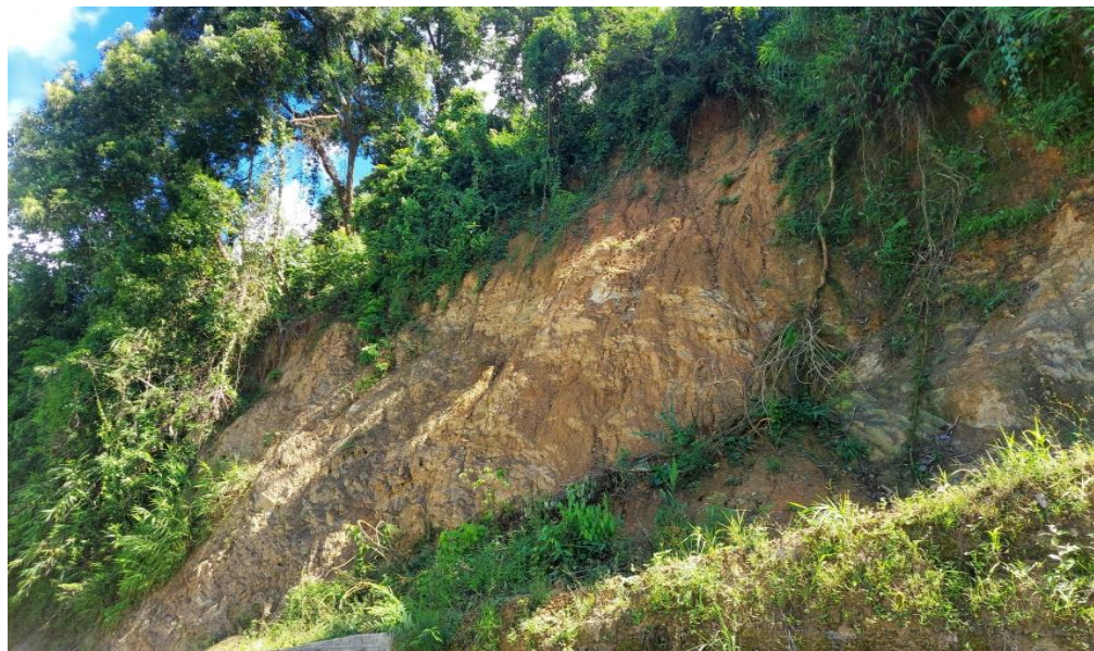
Location 10. Landslide (Translational type) near National highway, Aibawk.
