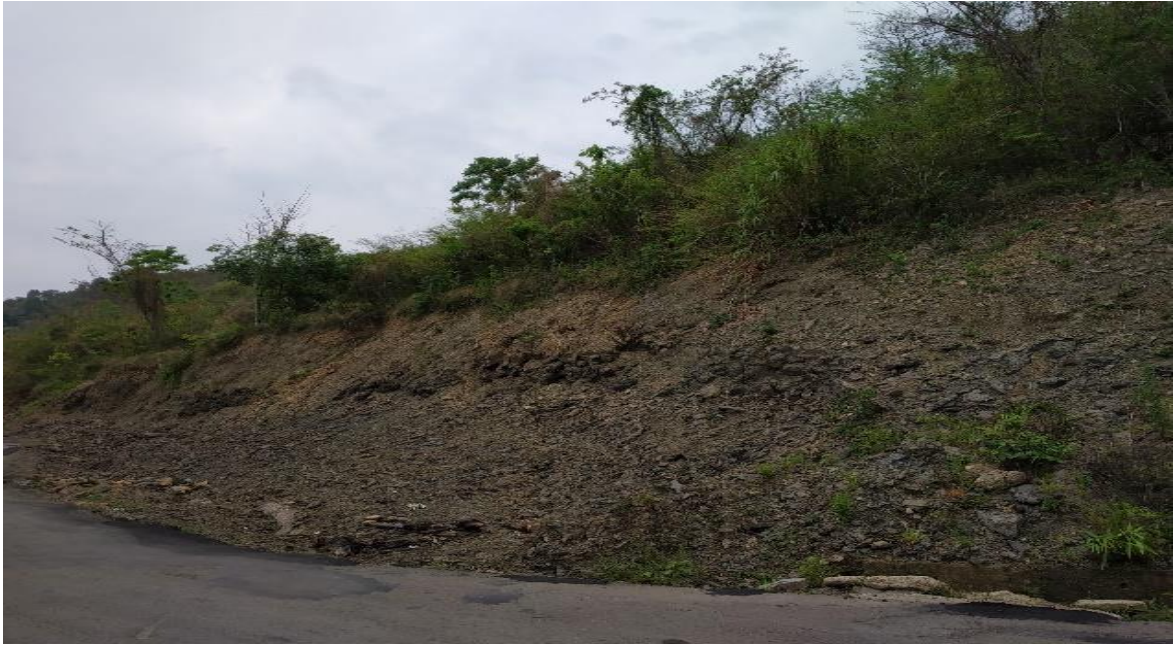
Location 3. Landslide (Translational type), Thiak,
