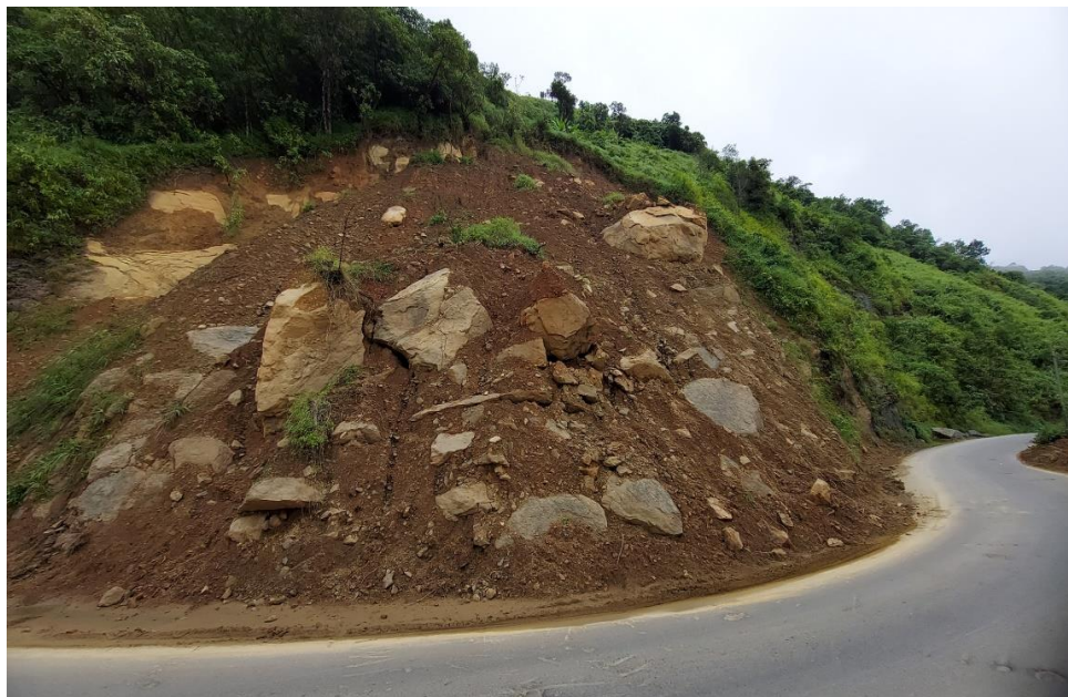
Location 12. Landslide (Translational type) near national highway, Hmuifang.
