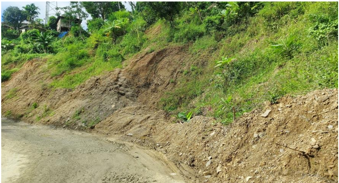
Location 6. Landslide (Translational type) near National highway, Hualngohmun.
