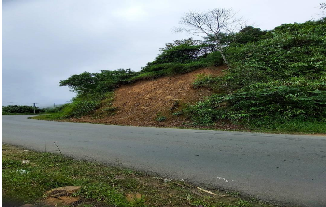
Location 13. Landslide (Translational type) near national highway, Hmuifang.
