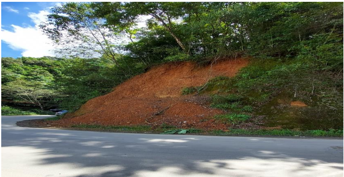
Location 18. Landslide (Translational type) near national highway, Sialsuk.
