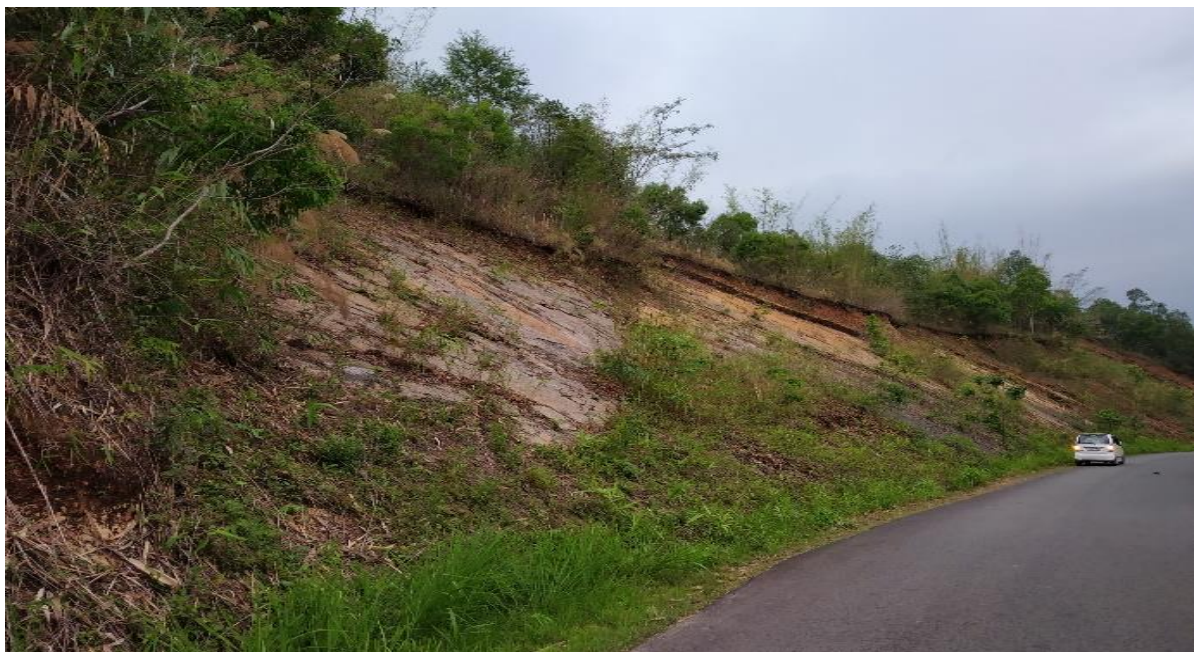
Location 4. Landslide (Translational type), Thiak 2.
