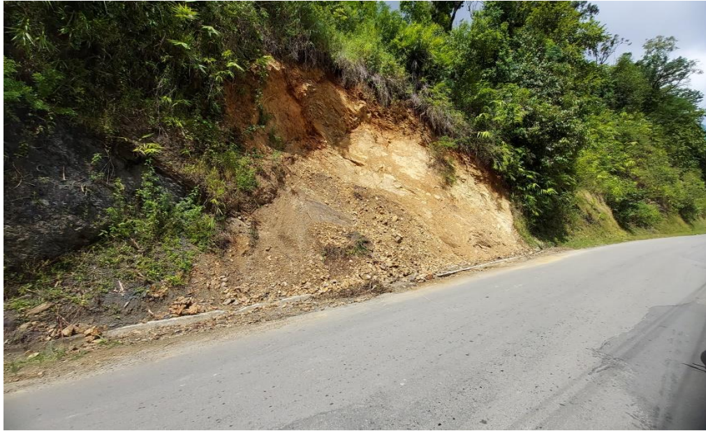
Location 15. Landslide (Translational type) near national highway, Sialsuk.
