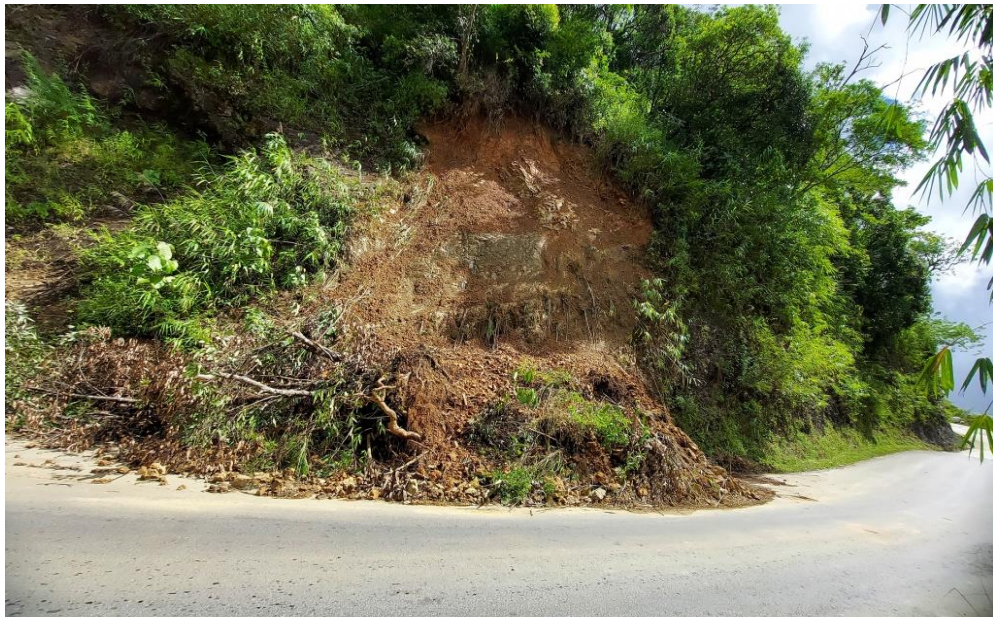
Location 16. Landslide (Debris slide) near national highway, Sialsuk.
