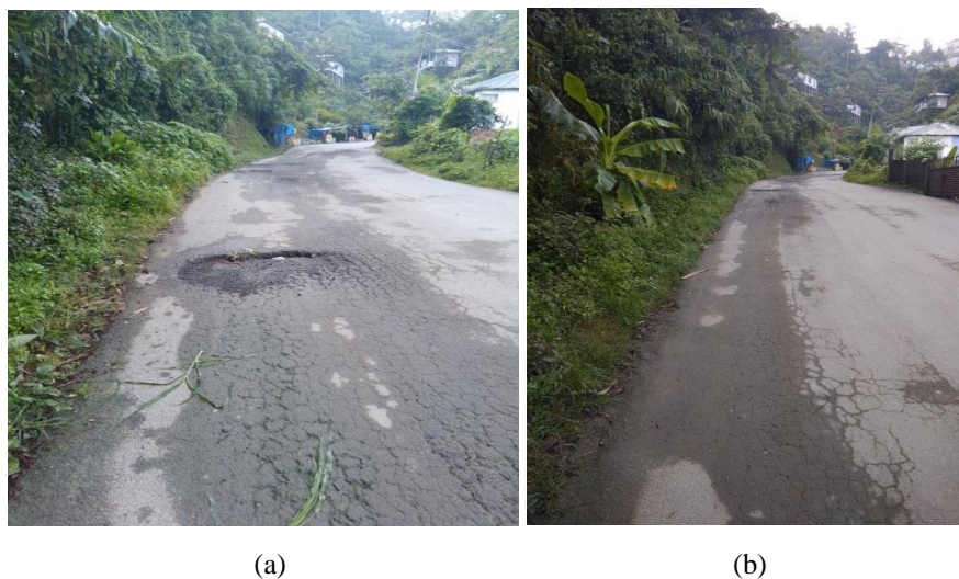
Fig. 4.6 (a) & (b) Elevated shoulder & tall grass obstructing surface drainage
