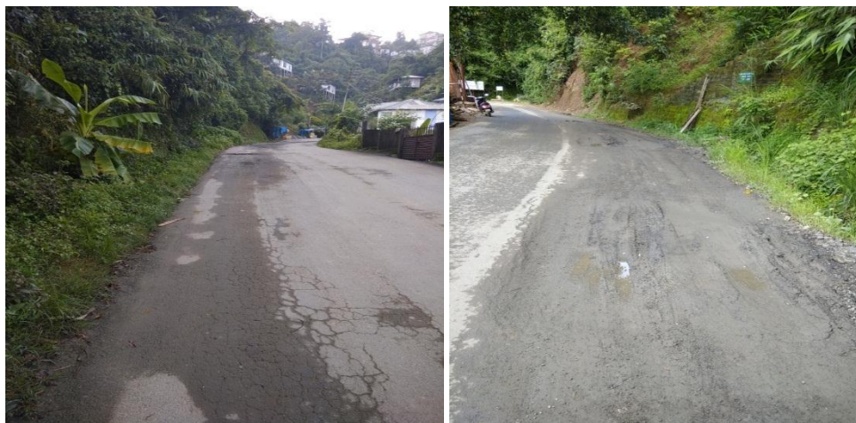
Fig.3.4 Raised shoulder and tall grass blocking surface drainage
