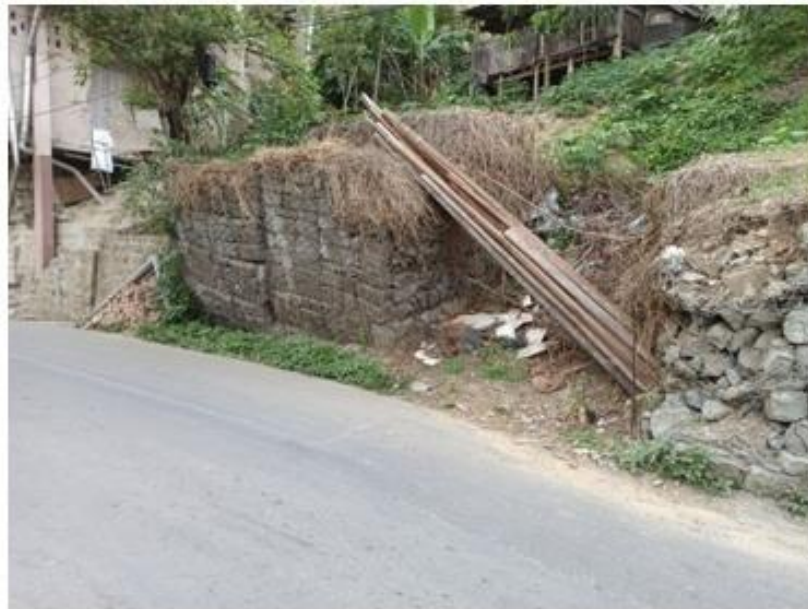
Figure: collapsed gabion wall
