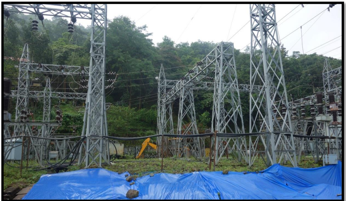
Figure 5.11. Zuangtui 132KV power substation
