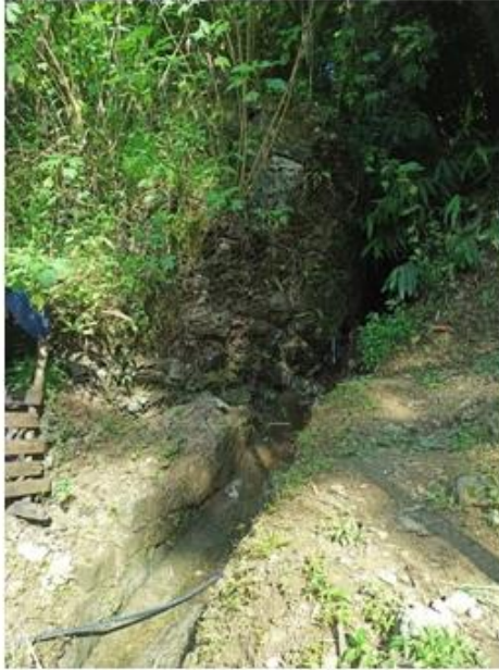
Figure: Bulging of gabion wall in location-1
