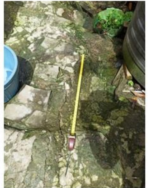
Figure: Fractures along private
