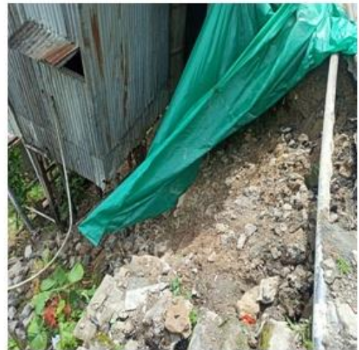
Figure: Collapsed of retaining wall
