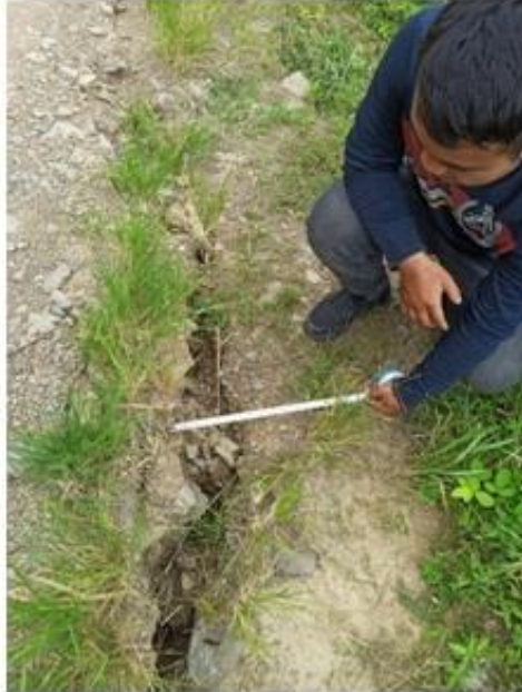
Figure: Cracks along the road
