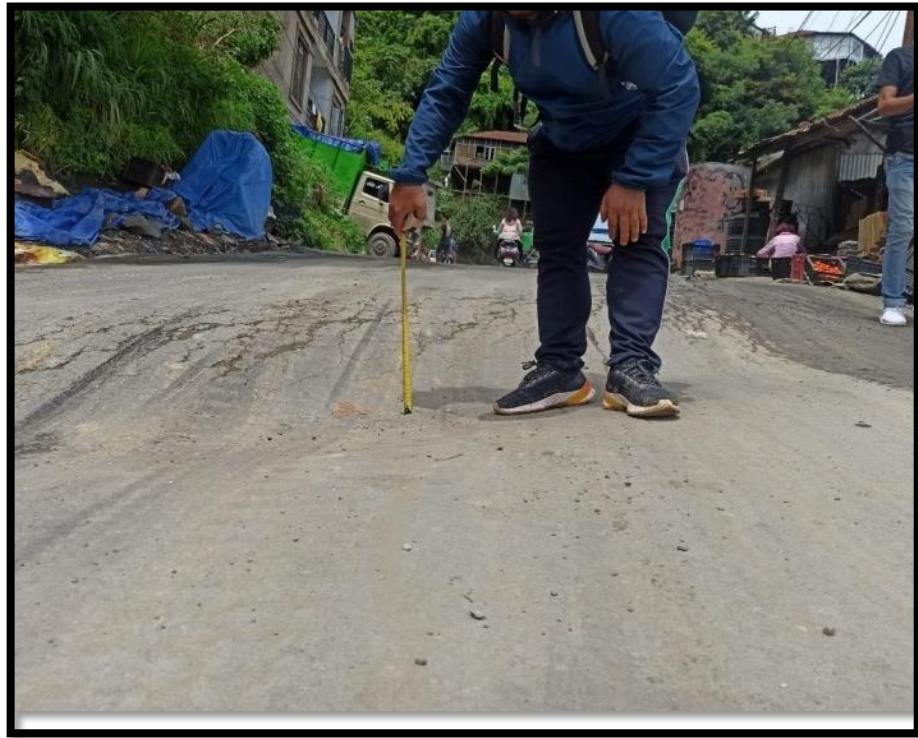
Figure 5.4. 1ft ground subsidence in location 1
