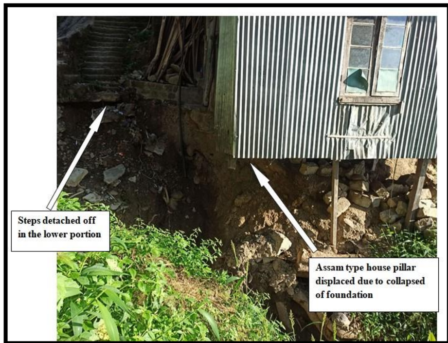
Figure 5.5. Collapsed of steps and building foundation
