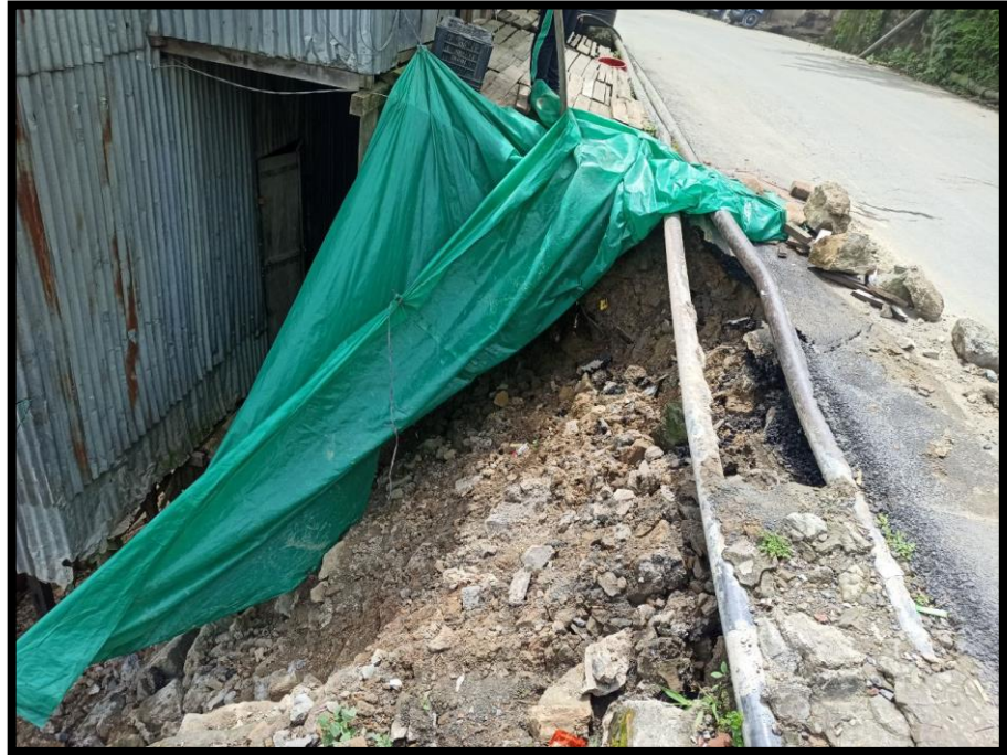
Figure 5.6. Collapsed of retaining wall
