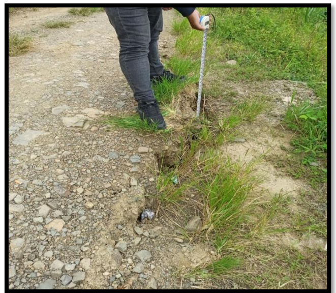
Figure 5.9. Tensional cracks observed in location-2
