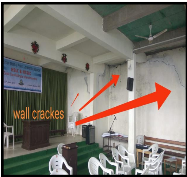
Figure 5.8. Cracks and fractures observed on the wall of Zuangtui Presbyterian Church
