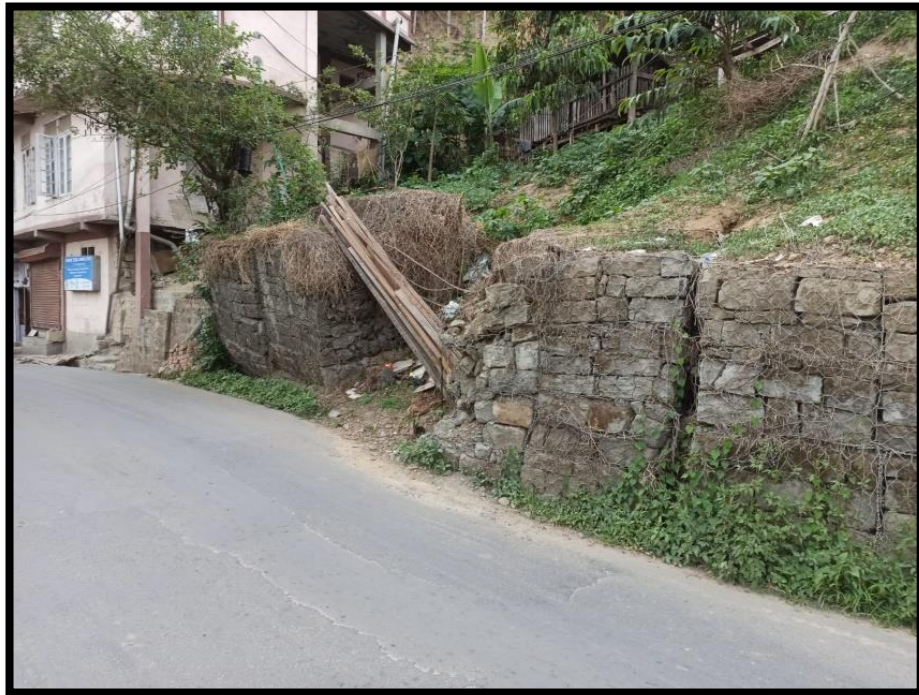
Figure 5.2. 6ft high gabion and masonry wall constructed in the upper portion of the study area
