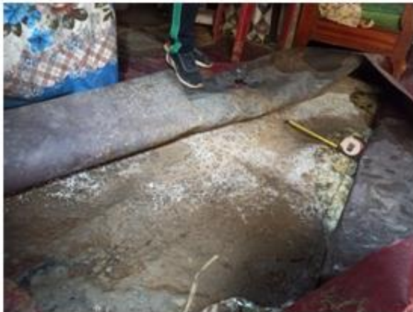
Figure: Cracks on the groundfloor of the house steps
