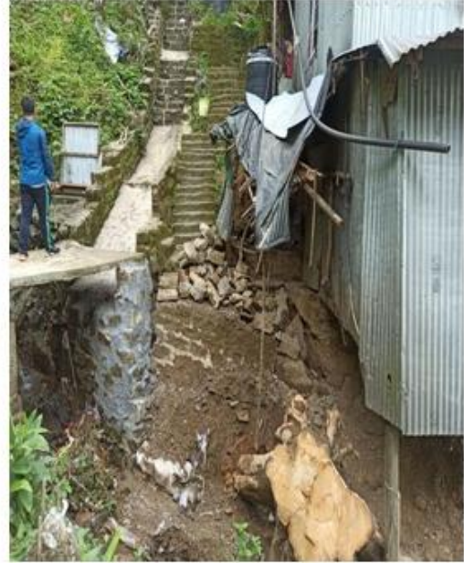
Figure: Collapsed of steps and pillar foundation
