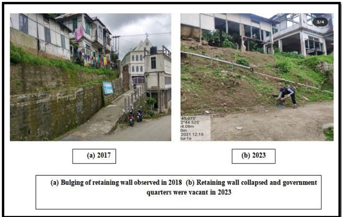
Figure 5.10. Collapsed Masonry retaining wall near Zuangtui Presbyterian Church
