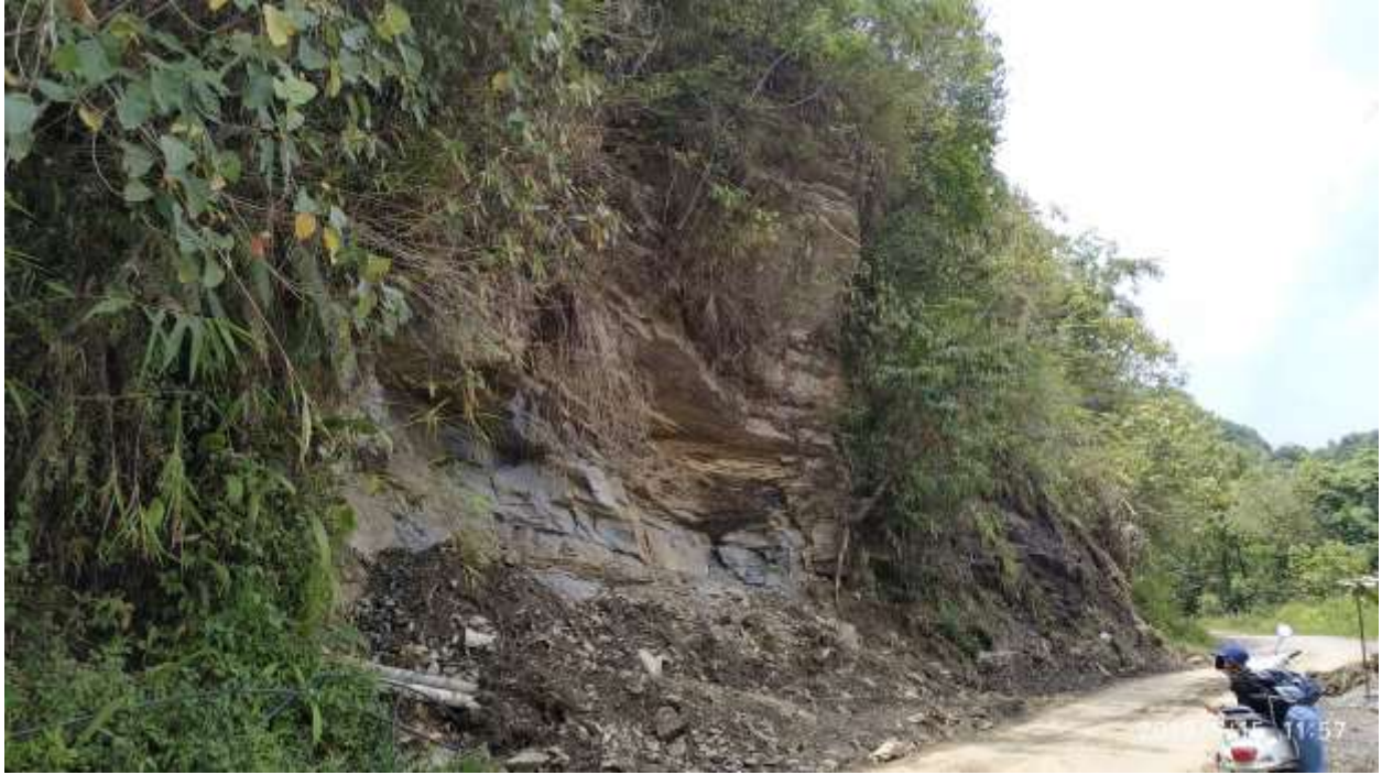
Location 3. Landslide (Rockfall), Tlungvel-1,
