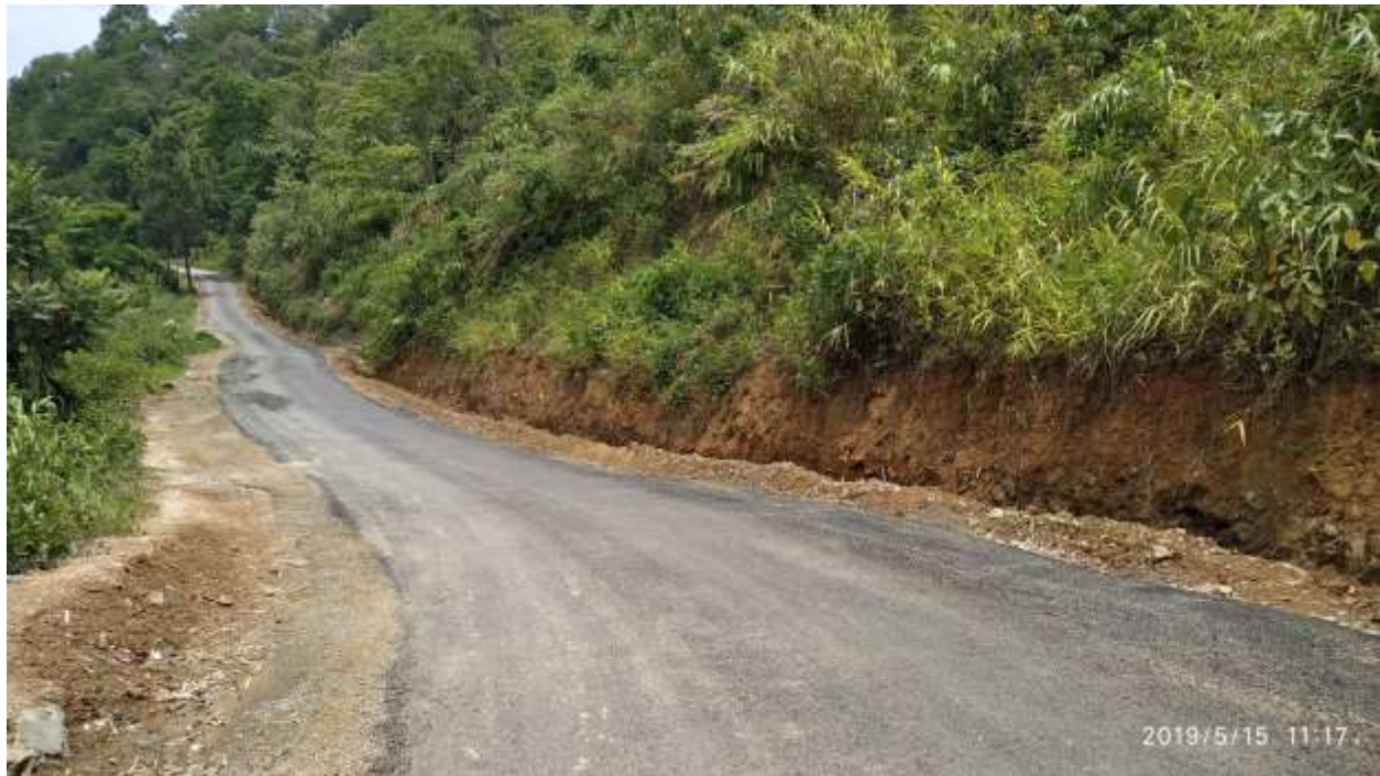
Landslide location 1. Landslide (Subsidence ), Phulmawi.
