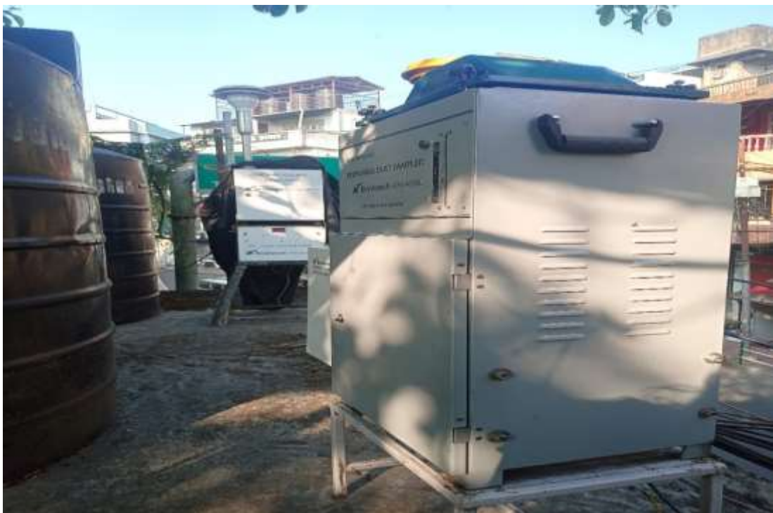
A-DP, (Dawrpui station)
