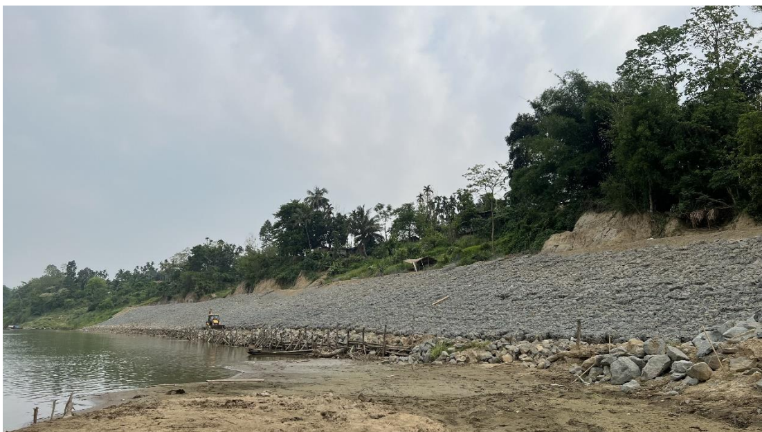
Figure 6.5 Embankment along Tlawng River in Bairabi
